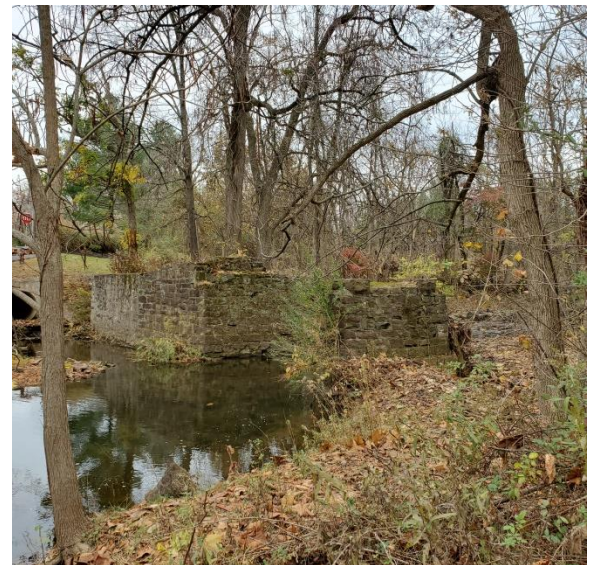
STONE PIERS FROM A FORMER TROLLEY BRIDGE ARE PROPOSED TO BE REPURPOSED FOR THE FROST LANE MULTI-USE TRAIL BRIDGE.
